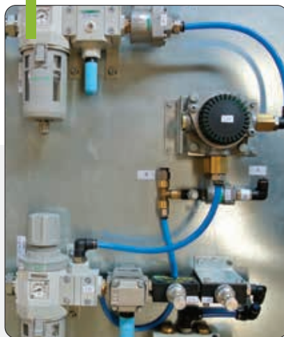
Winch pneumatic control panel
