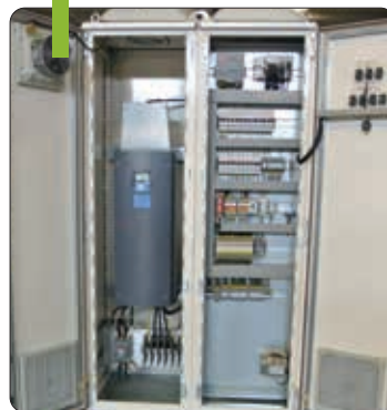
Winch control cabinet with frequency converter
